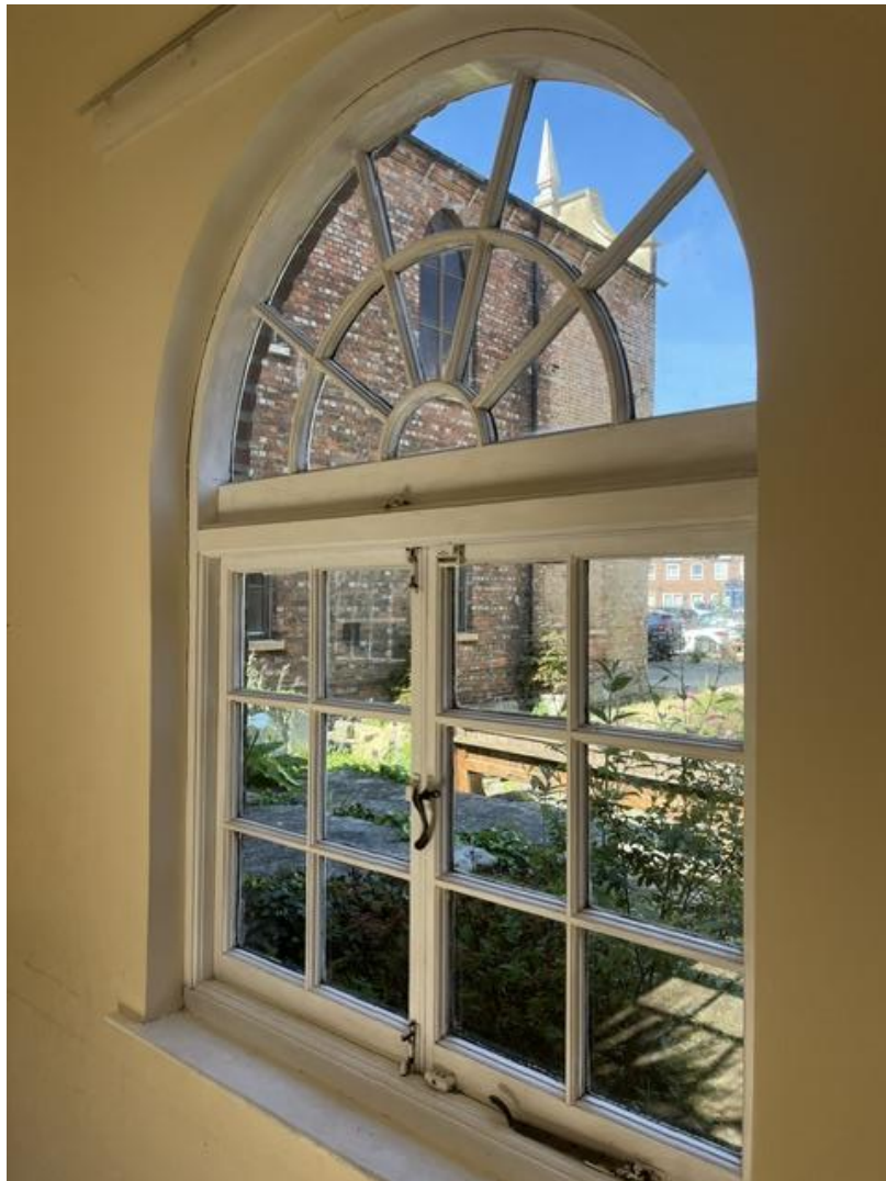
A view of the garden from the soon to be replaced/repared parlour window
